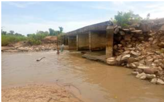
Plate 2: Flooded and Collapse Bridge at Kanikoko (Derived Savanna Zone)
